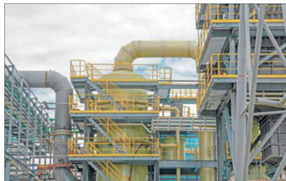
The modern production facility of sulfuric acid is set apart by its efficiency and environmental friendliness.
