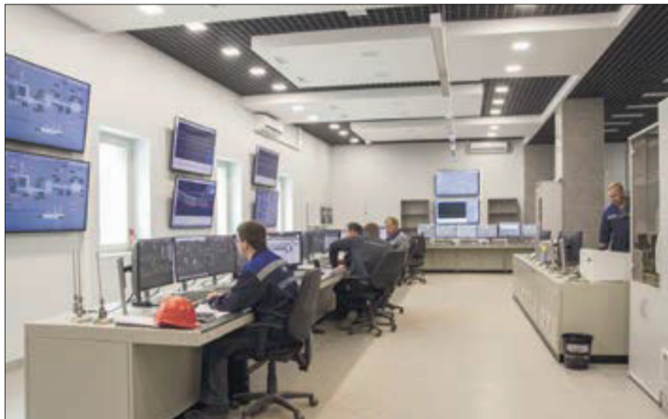
The central control panel of M-450/A-135 is preparing to start.
